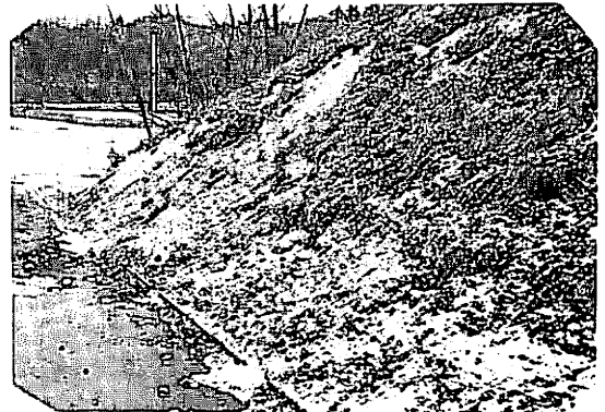
写真-3 凍害による切り取り斜面の崩壊 Photo.3 Failure of the cutting slope due to frost damage.
