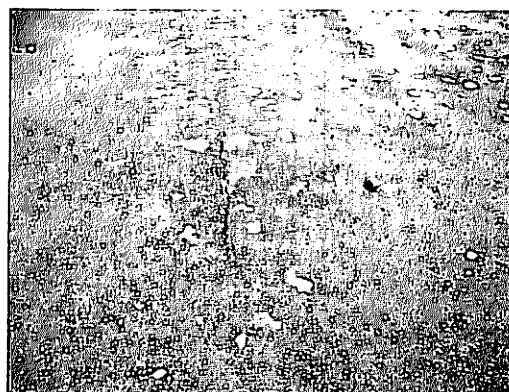
写真-3 き裂が生じた舗装 (Y工区) Photo.3 Cracks in pavement (Y experimental site)
