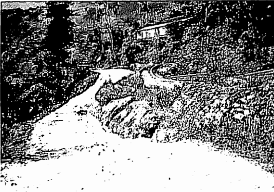
Photo 5 : View of Deflection of Road and Pipeline due to Landslide along Kathmandu-Trishuli Road. The Road was Straight before Landslide.
