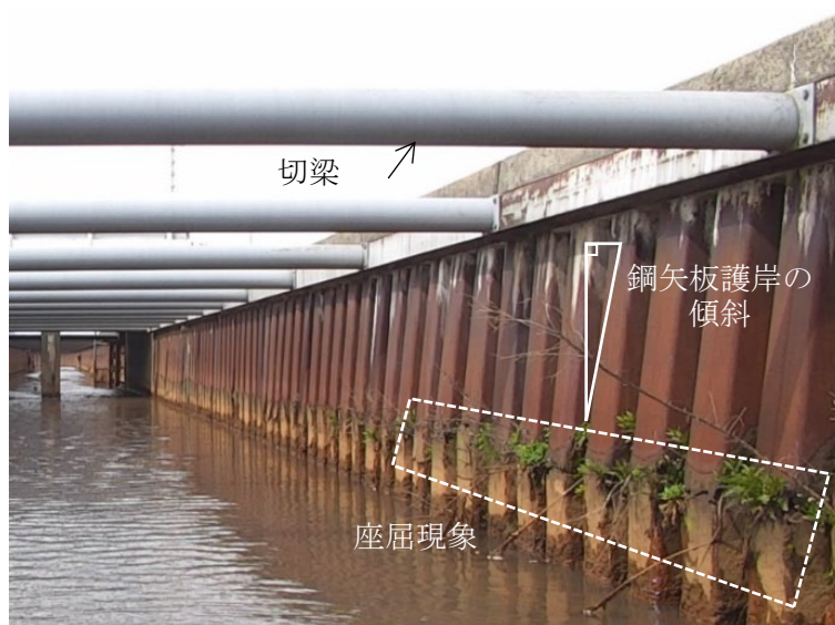
(a) 鋼矢板護岸の傾斜
