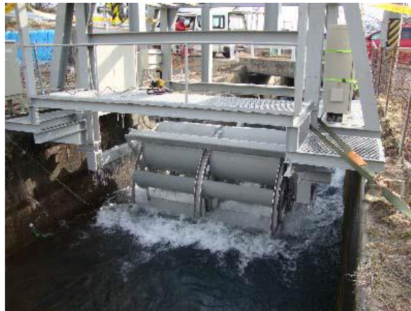
Fig.1-4 The horizontal application of the cross-flow hydraulic turbine (Ministry of Agriculture, Forestry and Fisheries).
